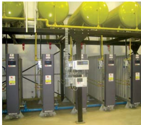
A six bank MAXIGAS installation. (Five generators in view) satisfy the peak demand, each capable of supplying 20% of the output. The banks cascade on and off load as the flow varies with factory production requirements. This saves significant energy costs during low flow periods, in the form of lower compressed air demand. The sixth bank provides 100% back-up and allows for 100% up-time during maintenance.
