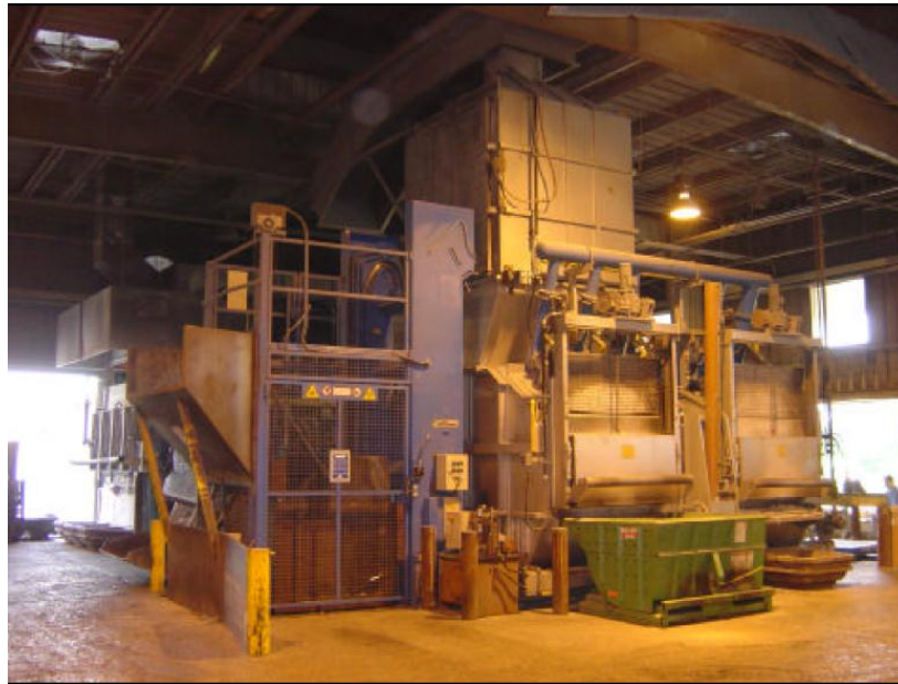
Figure 10 Tower aluminum melting furnace at Spartan Light Metal
