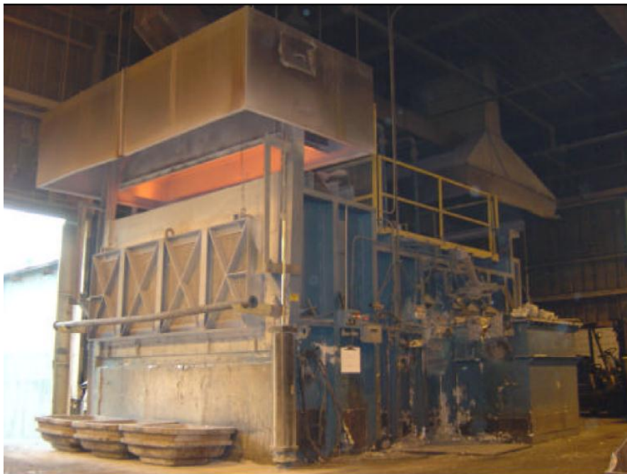
Figure 13 Reverberatory melting and holding furnace at Spartan Light Metal Products
