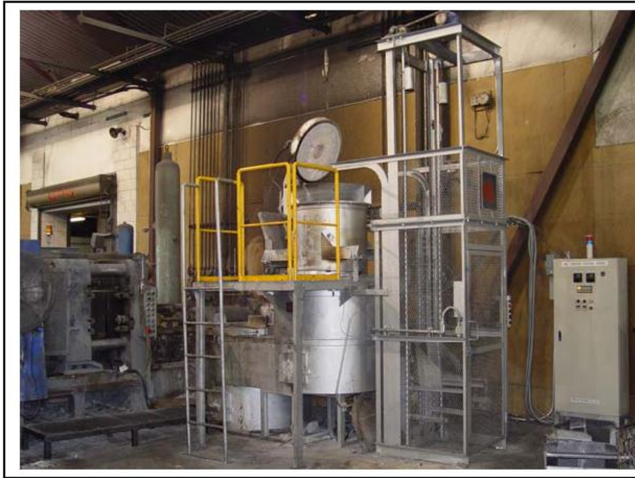
Figure 20 The Nikkan dual-crucible tower aluminum melting and holding furnace at Pressure Cast Products in Oakland, California
