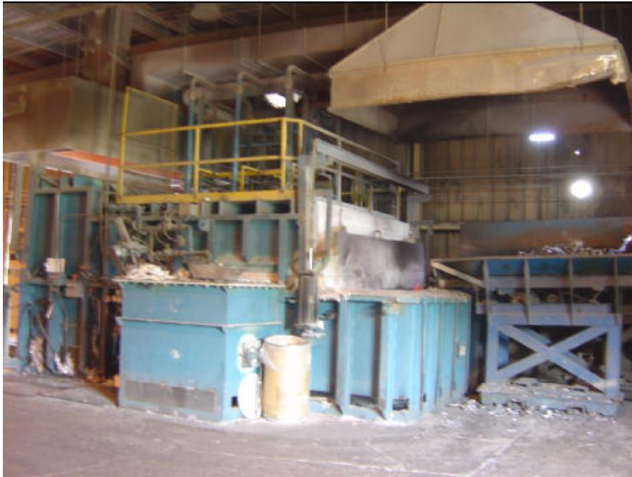
Figure 14 Vibrating chute for charging cold scrap into the well (right side)
